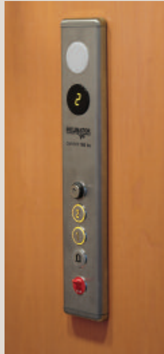
Car Control Station
